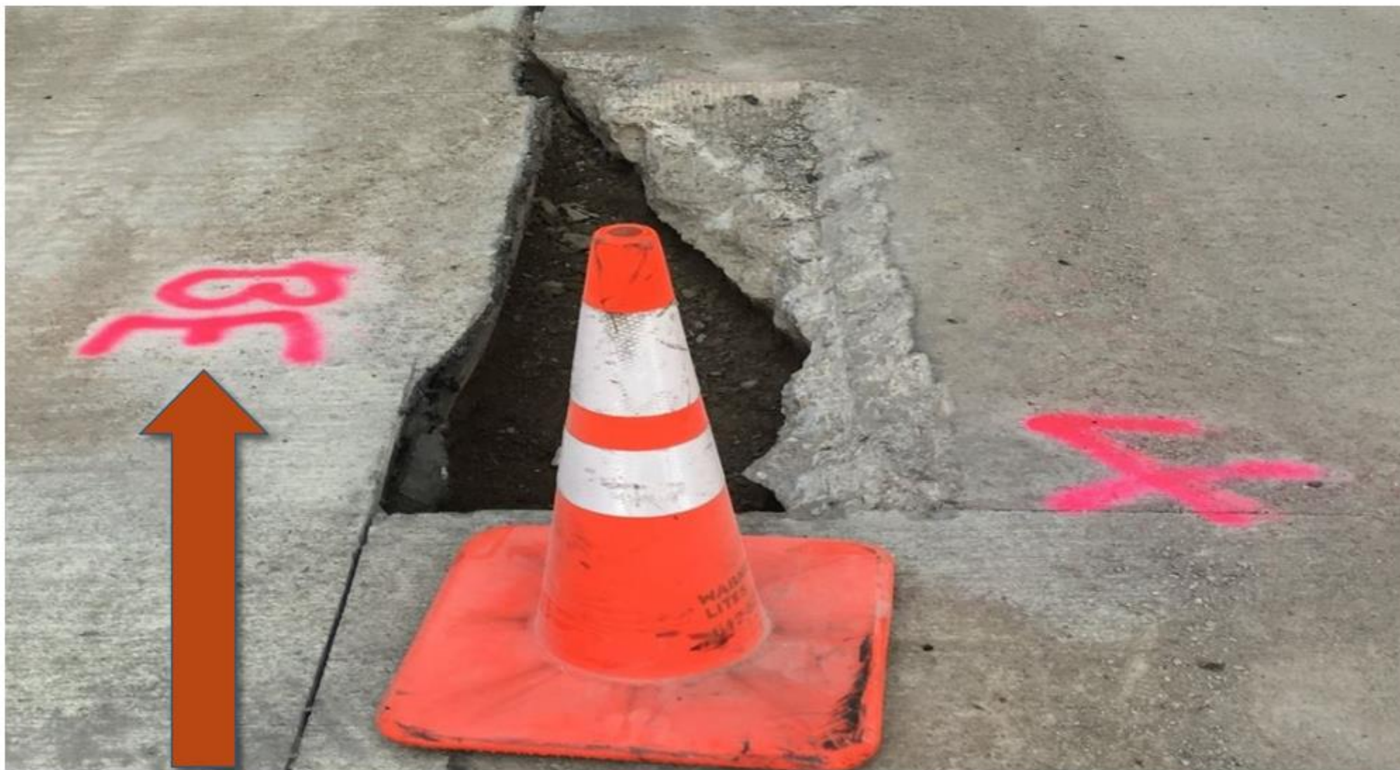
By marking "BE" on the pavement, the Inspector is instructing the Contractor to drill and grout 8-inch long No. 4 rebars (BE bars)
