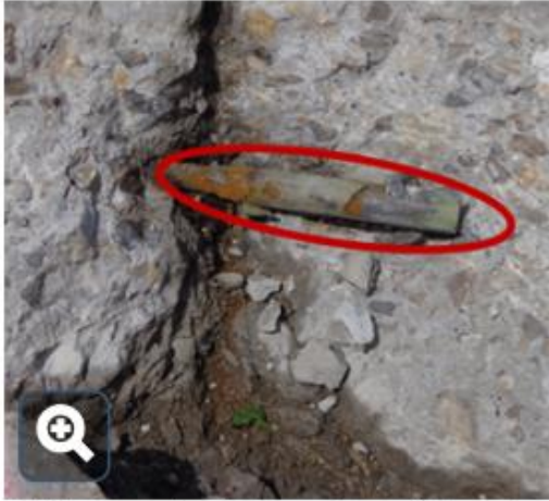
If the end of the dowel bar is exposed, remove the dowel bar (indicated by circle)
