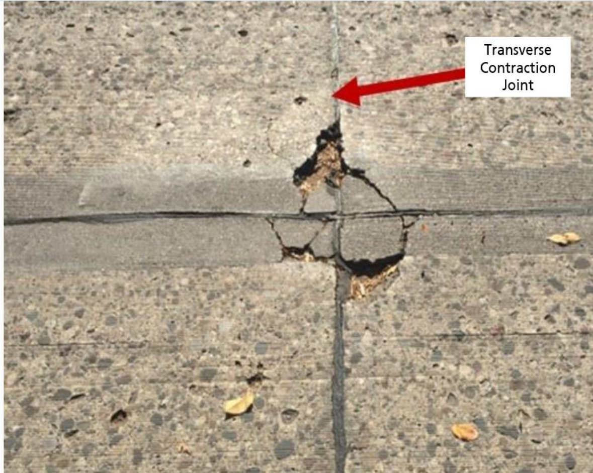
Compression relief not installed at time of construction resulted in compression failure (Picture taken 1 year after installation)
