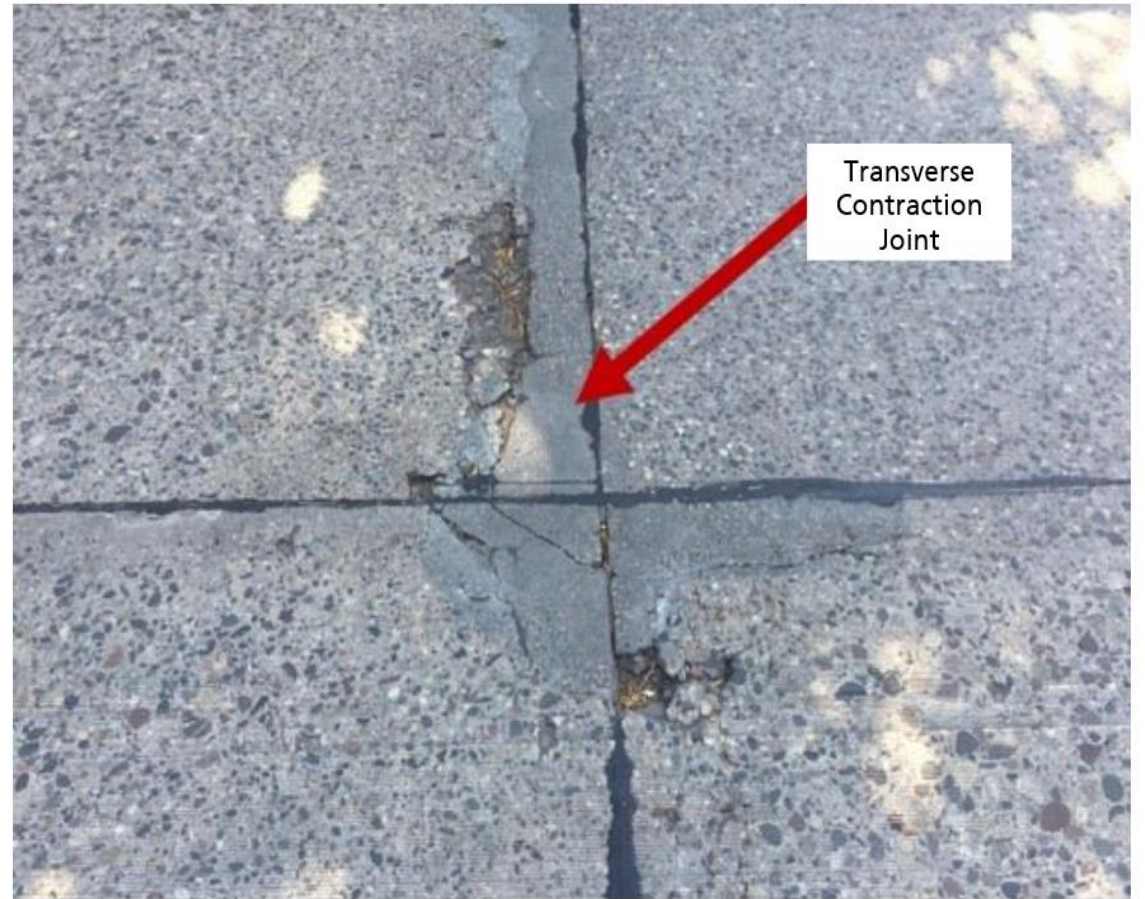
Compression relief not installed at time of construction resulted in compression failure (Picture taken 1 year after installation)
